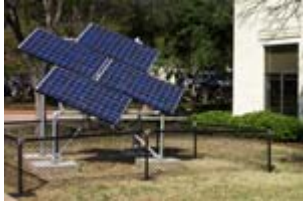
Dallas Museum of Nature & Science Solar Installation
